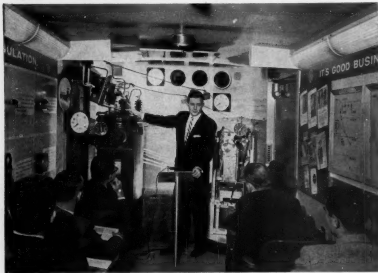
Inside of the Voltage Van, operated by the Voltage Regulator Product Section of General Electric Co. Equipment includes a fully operating ML32 regulator and equipment to demonstrate line drop compensation.
